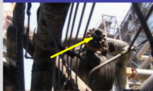
Figure 1. Carbon steel RHU heat exchanger outlet pipe (arrow) ruptured after operating only 3 months in high-temperature hydrogen service.
