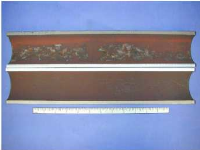
Figure 4-99 – I.D. deposits on CS boiler tube with damage due to caustic corrosion.
