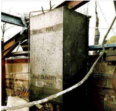
d) Diesel tank in pump house
