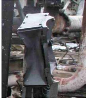
a) Crushed electrical connection box
